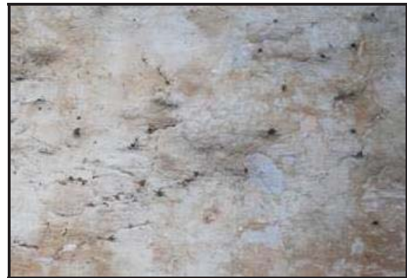
Peeling of plaster
