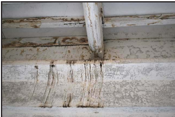
Seepage on wall and decayed wooden beam
