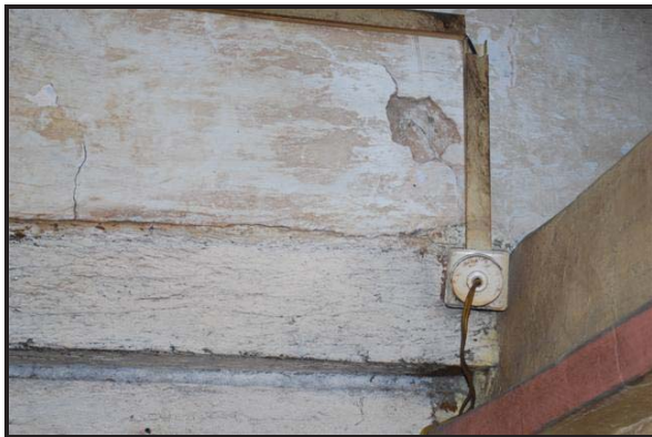
Open electric wiring
