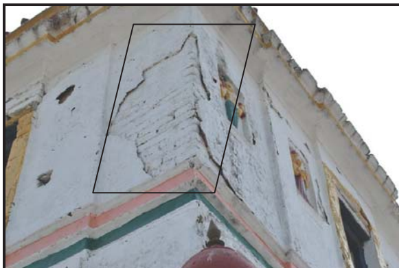
Loss of plaster
