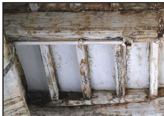
Decayed wooden beam and seepage on wall
