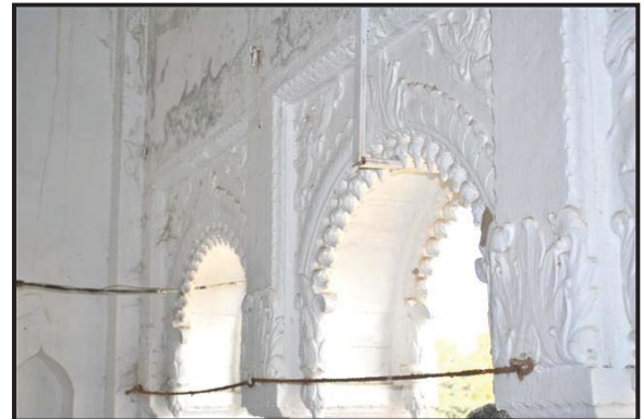
White wash on stucco and on relief work
